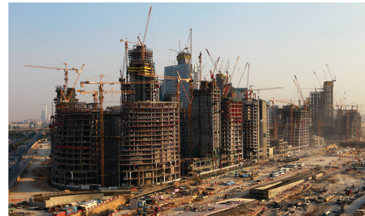
King Abdullah Financial District development, Riyadh, Saudi Arabia 80% Perimeter Barrier Edge supplied by SIDERISE
